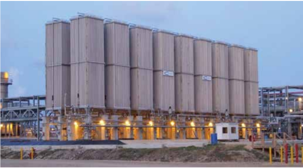
Figure 2. Send-out ambient vaporizer train at Cheniere's Sabine Pass LNG terminal.
