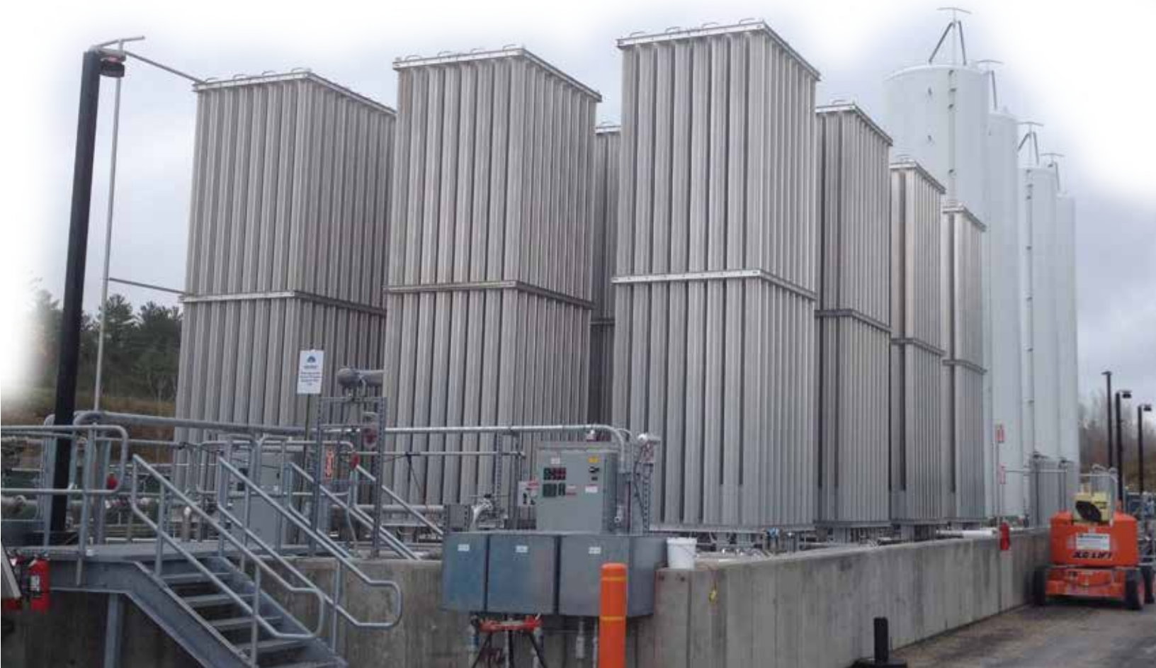
Figure 4. Satellite LNG ambientvaporizer system for industrial heat and power in the Northeastern U.S.
