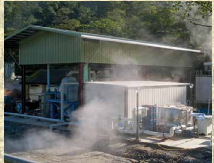
Figure 3 Geothermal Plant Operating at Qingshui, Taiwan with Microsteam® Turbine
