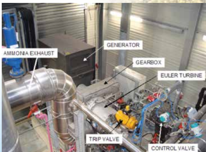
Figure 4 Euler Turbine Generator Operating in Geothermal Power Plant
