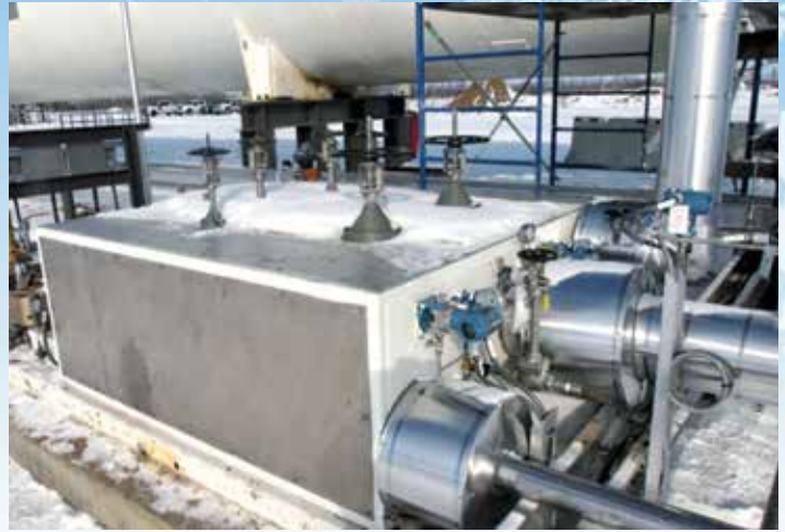
Dual LIN Pump Skid On Cosmodyne's Open Loop Plant Installation
